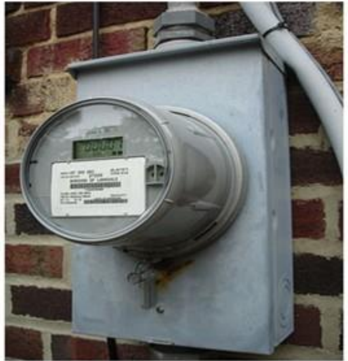
Older US residential electric meter location, retrofitted with a 1-phase digital smart meter. The meter communicates to its collection point using 900 MHz mesh network topology.
